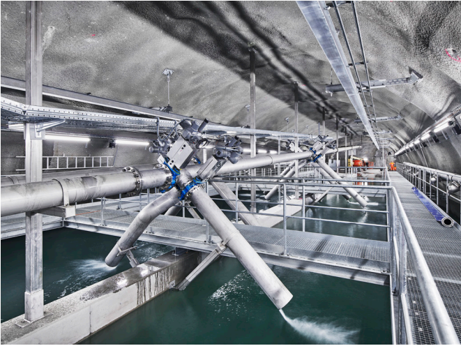
StreamLED 2: Customer / installation engineer: BLS Netz AG EPRO TRAFFIC GmbH: Electrical engineer
